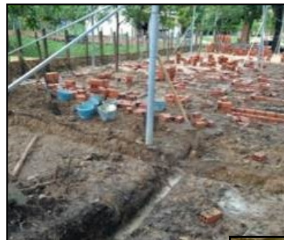
We constructed an outdoor classroom with shade covering, stove, and 42 seats in Siem Reap, Cambodia.
